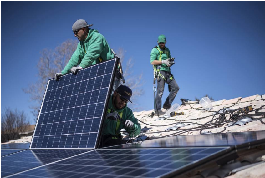
Workers doing a rooftop installation for SolarCity in Albuquerque, N.M., last month. PHOTO: SERGIO FLORES/BLOOMBERG NEWS
